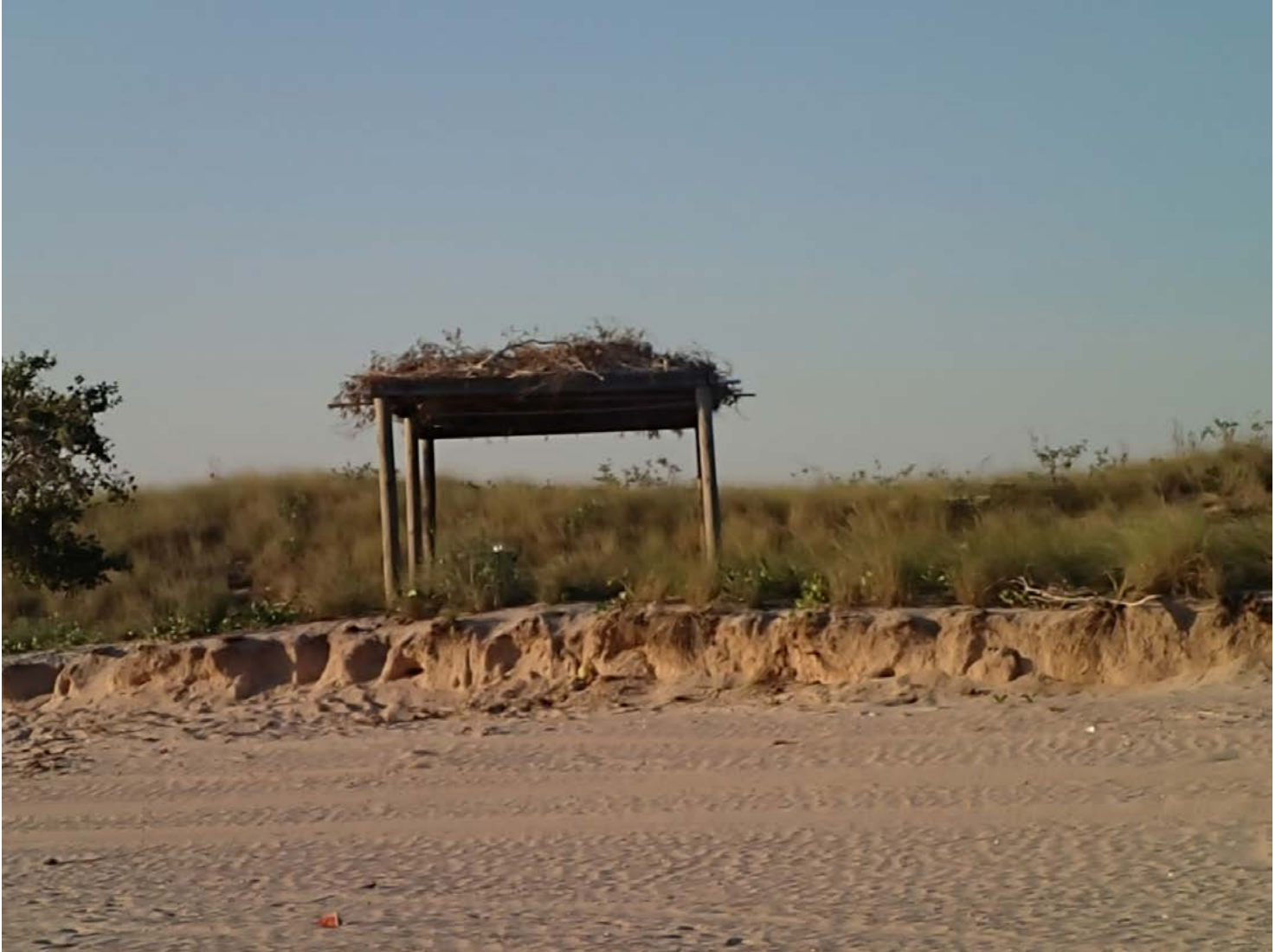
Figure 12 Coastal erosion from sea level rise has already claimed one bough shed at Whistle Creek. The remaining one shown here is clearly also under threat from coastal erosion.
