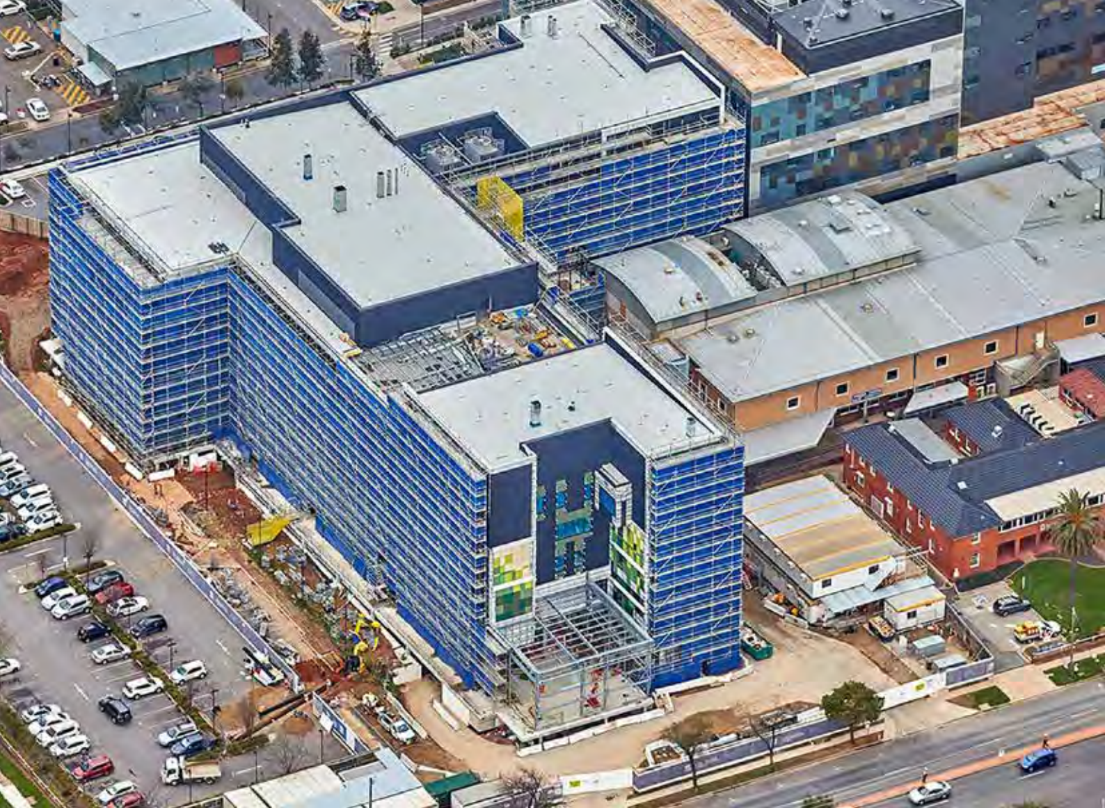
PHOTO: An aerial view from the corner of Edward and Docker streets in Wagga Wagga showing work on the façade of the new Stage 3 building.
